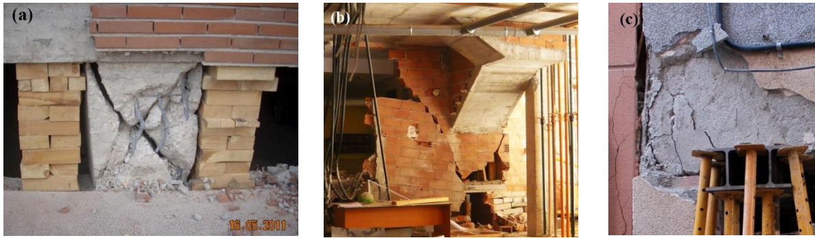
Figure 9. Brittle failure of “squat” column (a) (Vidal et al. 2011), masonry staircase (b), beam-column joint (c).
