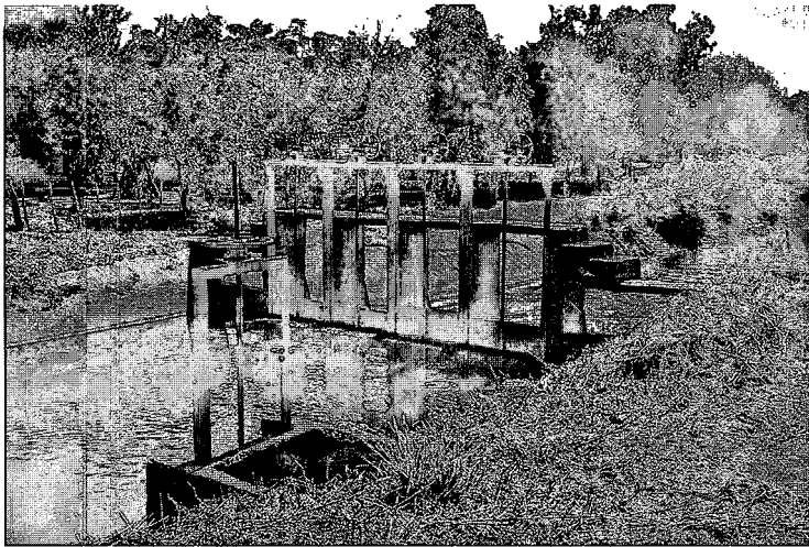
Photo 15 A new cross-regulator
