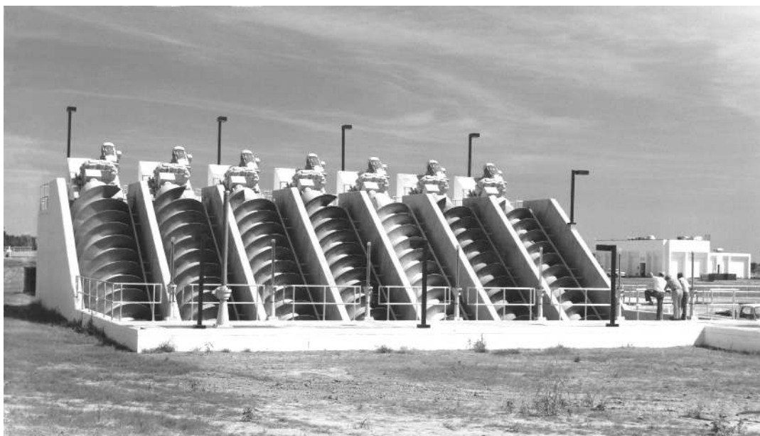
FIG. 4. Seven 96-Inch-Diameter, 3-Flight Screw Pumps That Lift Wastewater from Pretreatment Section to Balance of Treatment Plant in Memphis, Tenn. [Each Pump Has Capacity of 19,900 gal./min (Courtesy Lakeside Equipment Corp., Bartlett, Ill.)]
