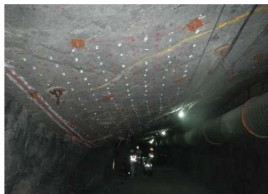
Figure 5—Hangingwall survey block at Mine B. The grid of white spray paint markings was used to guide data acquisition
