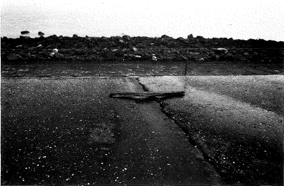
Photo 29 Because of a poorly constructed daily joint the subsoil material has been washed out causing the revetment material to deform
