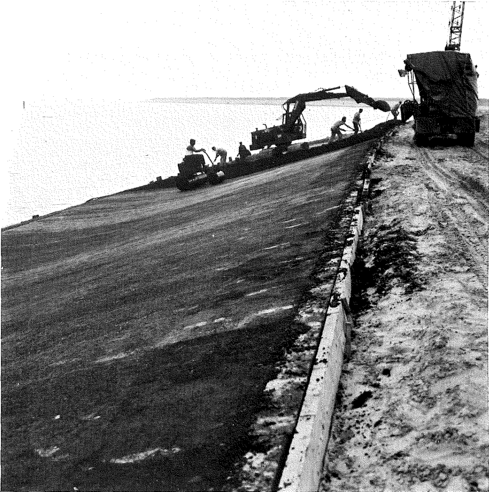
Photo 10 Construction of an asphaltic concrete revetment: The crane dumps the asphalt on the slope; the backhoe spreads the asphalt
