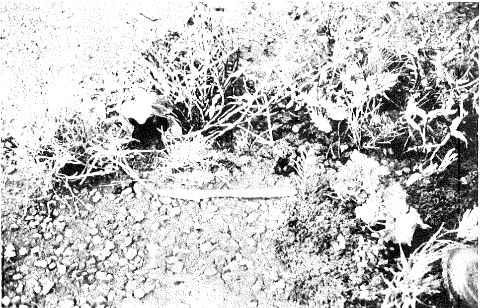
Photo 2 Plant growth damaging an asphaltic concrete revetment
