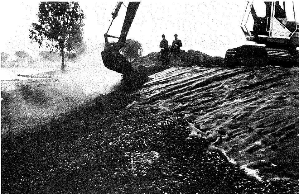
Photo 21 Placing an open stone asphalt layer on a filter cloth using a backhoe
