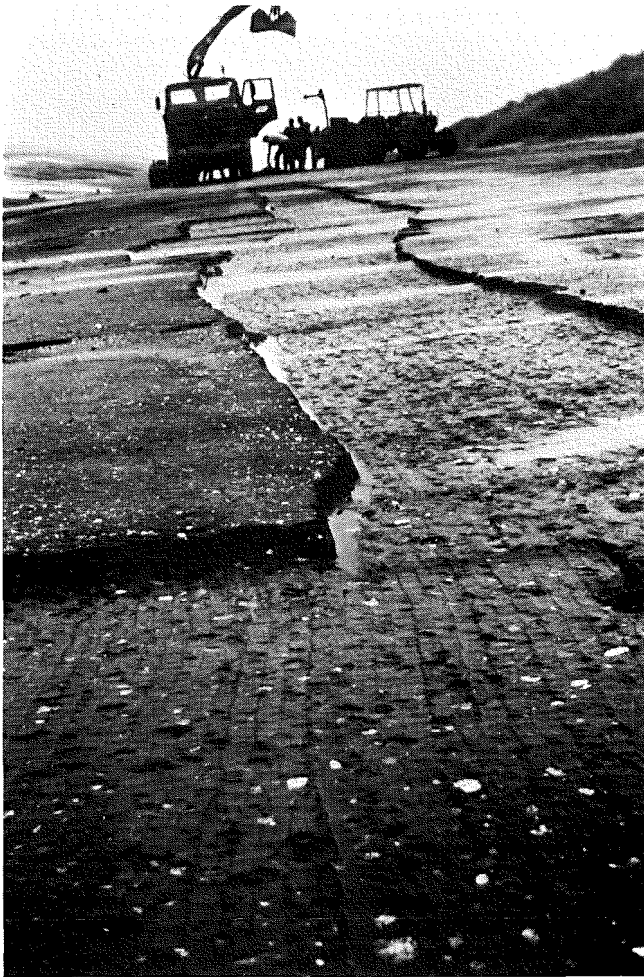
Photo 30 Repairing the seriously damaged surface of an asphaltic concrete revetment: The damaged area has been frayed out
