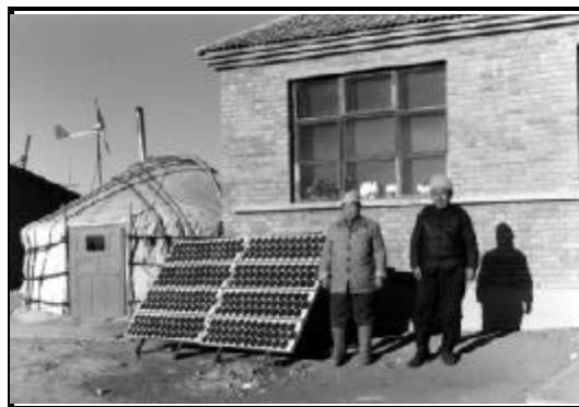
Figure 2. 500-Watt PV/wind hybrid household system in Inner Mongolia. Courtesy of Wang Sicheng, JiKe Company.
