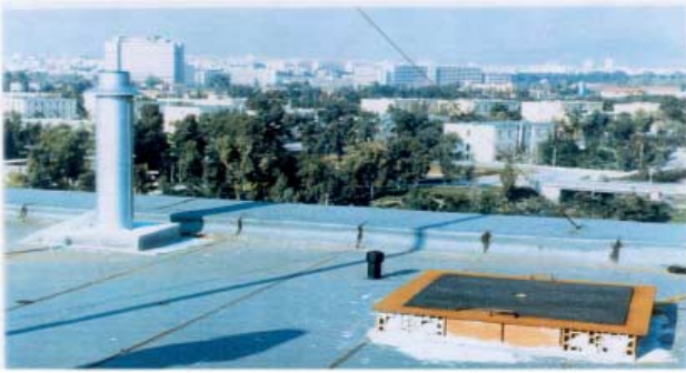
Fig. 1. The installation of the Disdrometer RD-69 on the roof of the Water Resources building.
