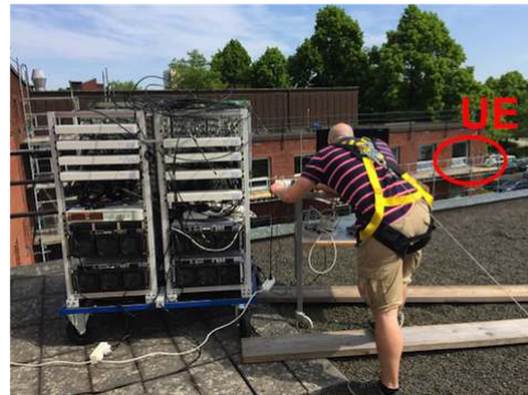
Fig. 14. The outdoor test scenario setup with the BS deployed on the rooftop of the department building marked with two UEs on the opposite building wing.
