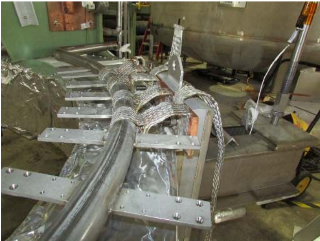
Fig. 2. The cooling pipe with welded tabs. One of the magnet supports can be seen to the right, and thermal intercept flexible straps can be seen at the center.
