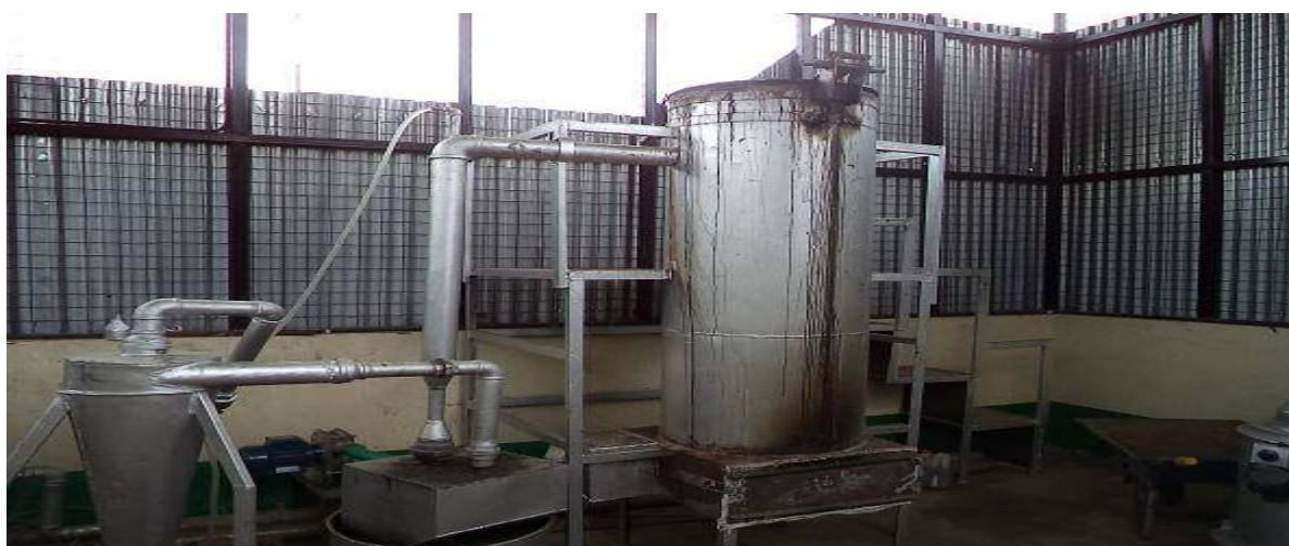
Figure 3. Gasifier in the Shed.
