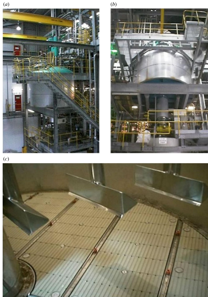
Figure 1. Views of the 36 m 3 ProceMon pressure filter; (a) and (b) external views and (c) internal view showing agitator blades and fixing bases for supporting the filter cloth.
