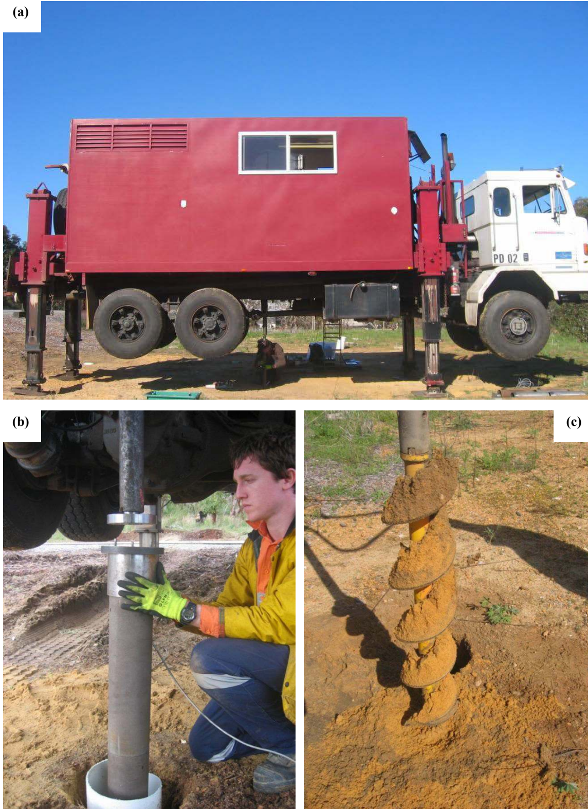
Figure 4.12. Pile installation: (a) CPT truck provides the reaction and jacking facilities; (b) pile head connection for efficient incremental jacking procedures; (c) preboring in phase 4 testings
