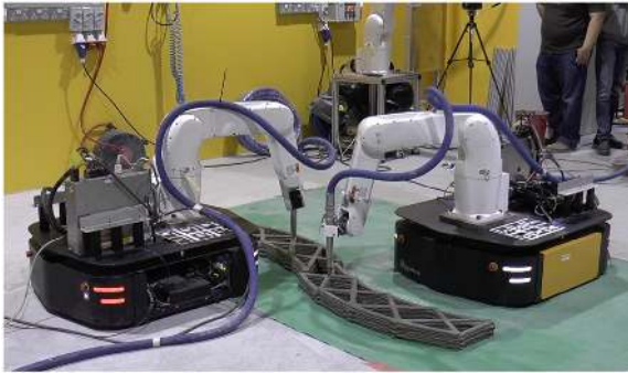
Fig. 1. Concurrent printing of a large, single-piece, concrete structure by two mobile robot printers. See the full video of the experiment at https://youtu.be/p_jcG25tUoo .
