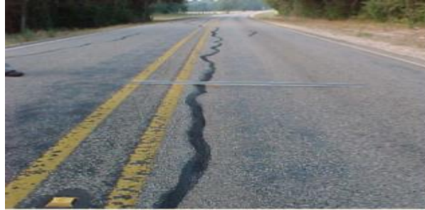
Figure 2. 9 Typical longitudinal crack developed on pavements over expansive clays (Zornberg et al. 2015)
