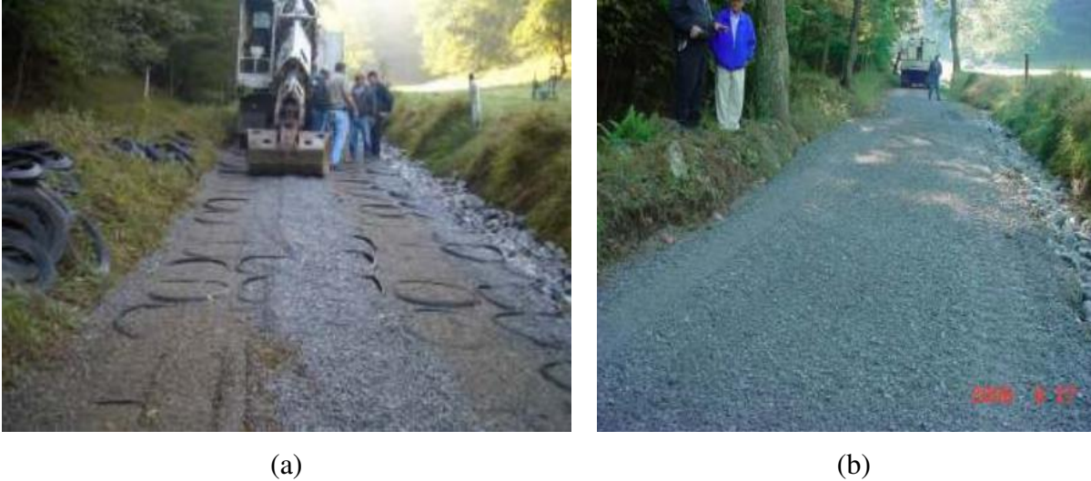
Figure 5. 2 (a) Mechanical concrete base in Doddridge County, WV (b) Wearing surface (Mechanical Concrete ® 2009)
