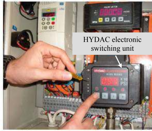
Figure 6-8 Setting the desired pressure in the hydraulic system switch located in the control panel.
