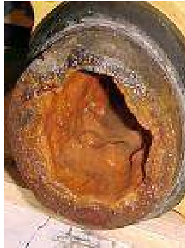
Biofilm on pipe
