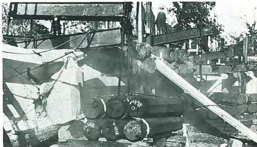
(b) Girder at moment of failure.
