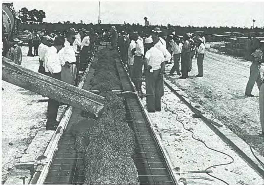
Fig. 29. Demonstrating the production of a 14-in. (356 mm) deep by 4-ft. (1.2 m) wide double-tee at R. H. Wright & Co., Fort Lauderdale, Florida. Note that this form used a steel liner for the stems only. The remainder of the form was concrete.
