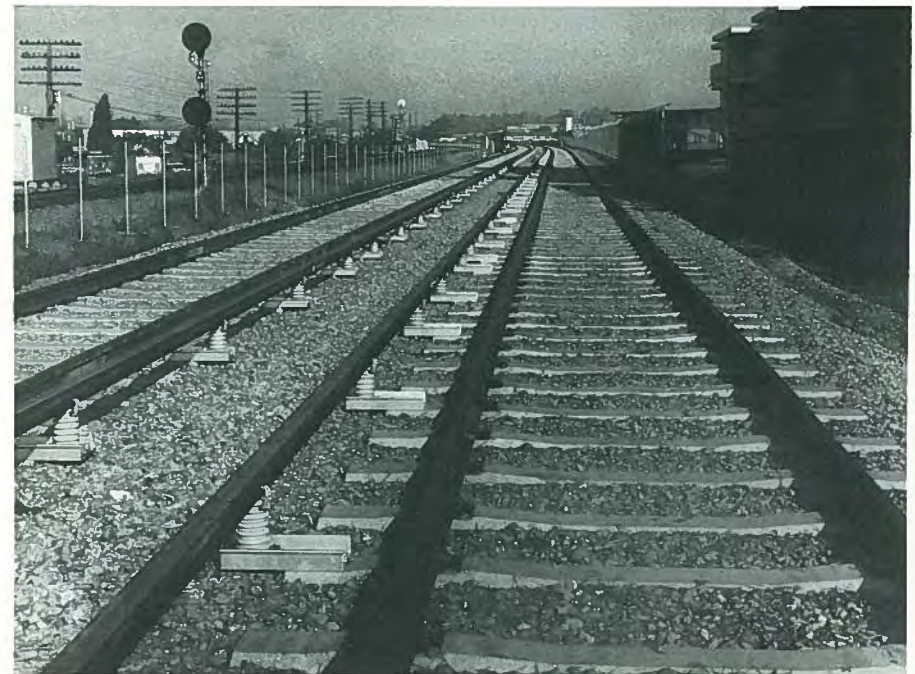
Fig. 53. Gerwick RT-2 type cross-ties as installed into Bart track system at Hayward, California.
