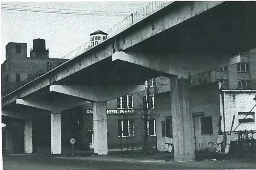
Fig. 23. In 1956, precast single-tee sections for a viaduct were made at Prestressed Concrete of Colorado's second pretensioning plant and transported to the site.
