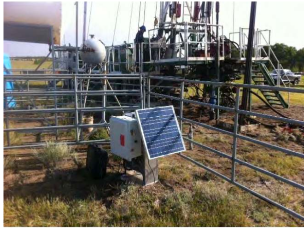
Figure 6.5. Ventmeter™ installed at a wellbore
