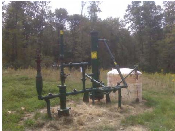
Figure 6.1. Dead vegetation surrounding a natural gas wellhead in Pennsylvania (Emily Grubet)
