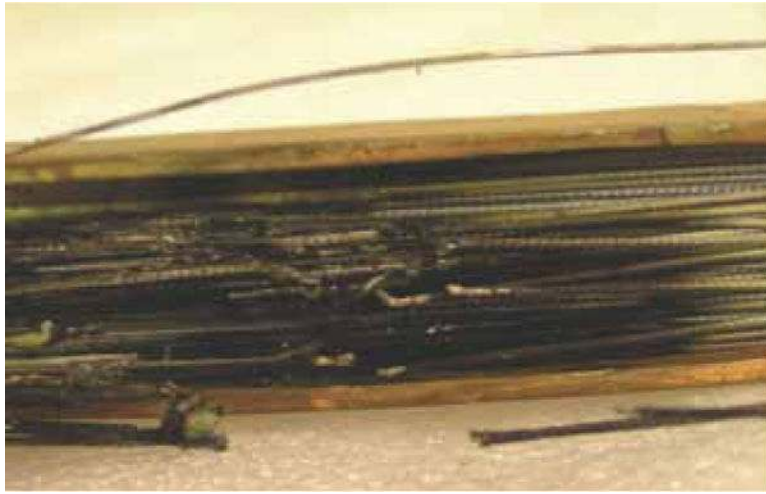
Fig. 7. Photo of a damaged top coil winding section after a premature quench at 79 A.
