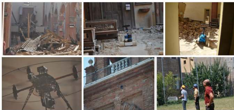
Fig. 2 Duomo in Mirandola, Northern Italy. Top: Main aisle (l.), UGV exploring eastern aisle (m.), top of the western aisle (r.). Bottom: UAV exploring eastern aisle (l.), exploring cracks in bell tower (m.), UAV team (r.).
