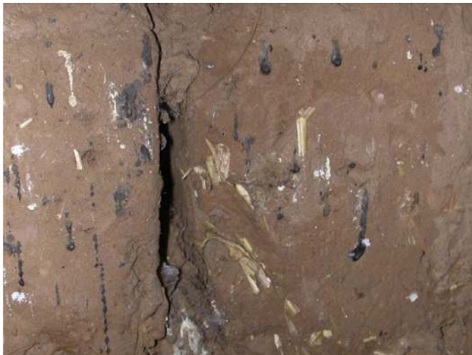
Figure 2. Crack offering refuge to triatomine bugs and fecal streaks in a mud wall. (A color version of this figure is available at www.vetres.org .)
