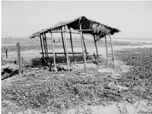
Fig. 6. Damaged hut in Kapyet Thuang Village.
