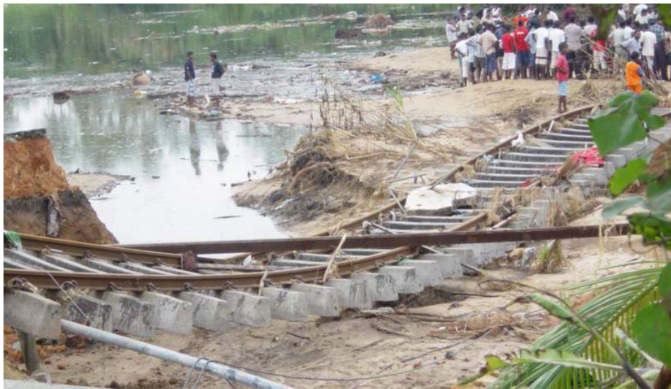
Figure 12. Heavily-damaged southern railway near Akurala.
