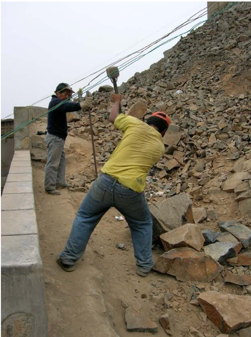
Two men breaking up rock that has been pried and sledge-hammered out of the hill. Usually, a retaining wall is built first, then rock is tumbled out from beside the wall to form the base of a road. Many of the access roads have been built in this fashion. Men often do the heavier work like that shown above. Excess rock is being broken up to be taken away in dump trucks. Photo: author
