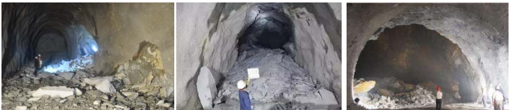
Fig. 6. Tunnels destruction cases along railway
