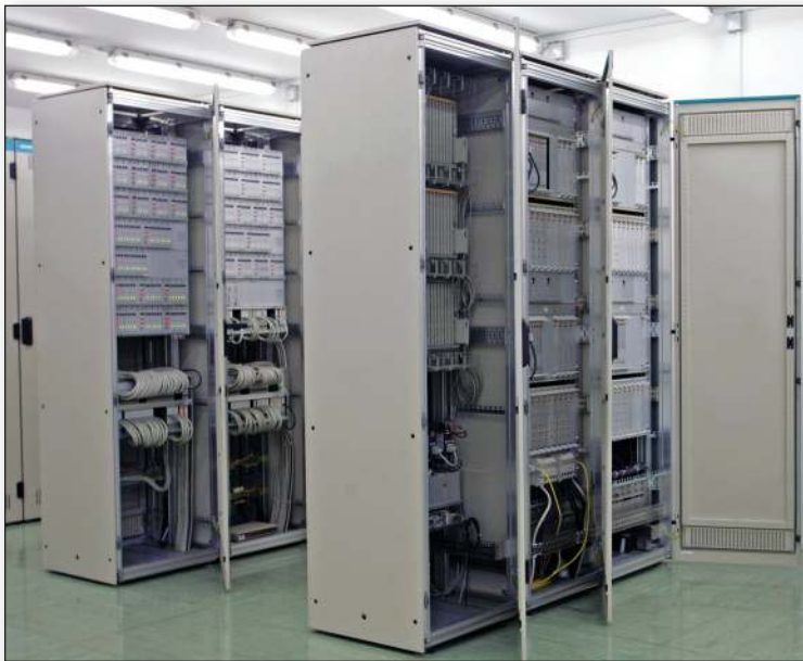
Figure 3. Railway Interlocking System Hardware.
