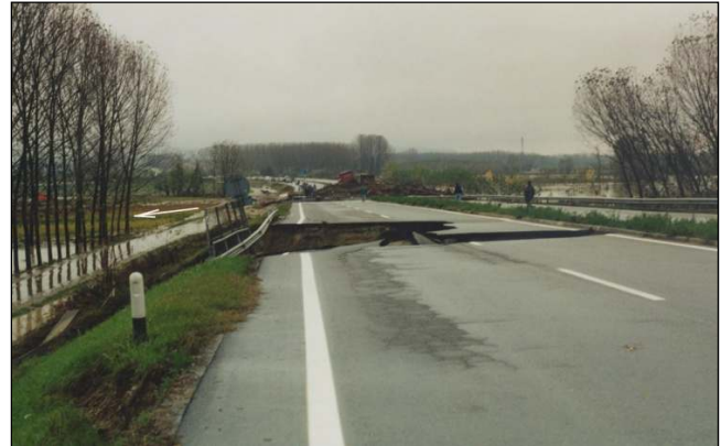
Fig. 14. A large failure caused by the undercutting floodwaters blocked the Asti-Cuneo Highway. In the background, the light subsidence of the highway where the waters overflowed (K in Fig. 2) left a large accumulation of uprooted trees.
