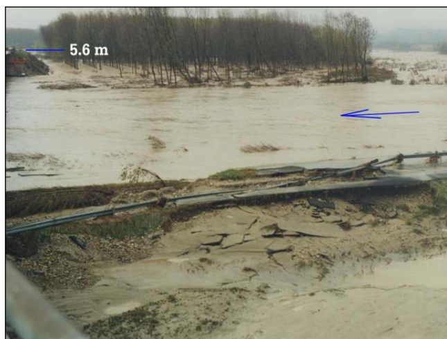
Fig. 3. 6 November 1994, 13:00 LT. The Tanaro River is still swollen. The effects of the flooding are evident. In the foreground, the link road of the Asti-Cuneo highway has been stripped by the violence of the waters. On the left, along the highway embankment, is the site where the deepest floodwaters (5.60 m) were measured (X in Fig. 2). In the background is a thick poplar forest recently planted in a natural area along the Tanaro.
