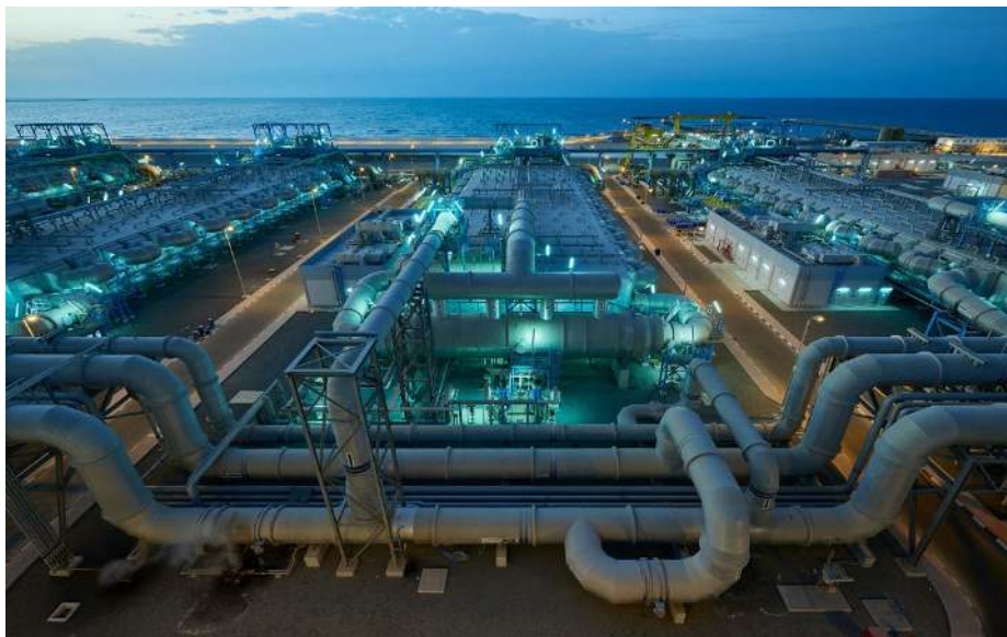
FIGURE 3. Dubai's huge desalination plant [56].
