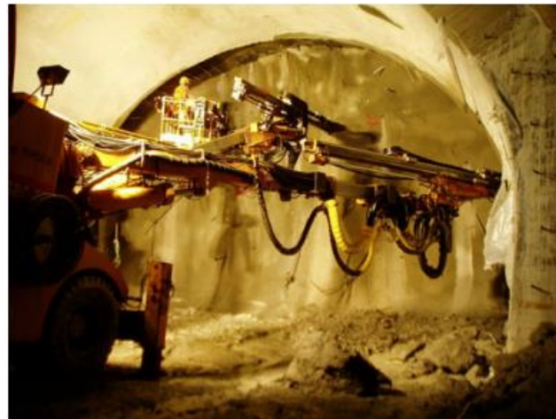
Figure 14. Collapse of the working face of Atlantic Ocean tunnel [87].
