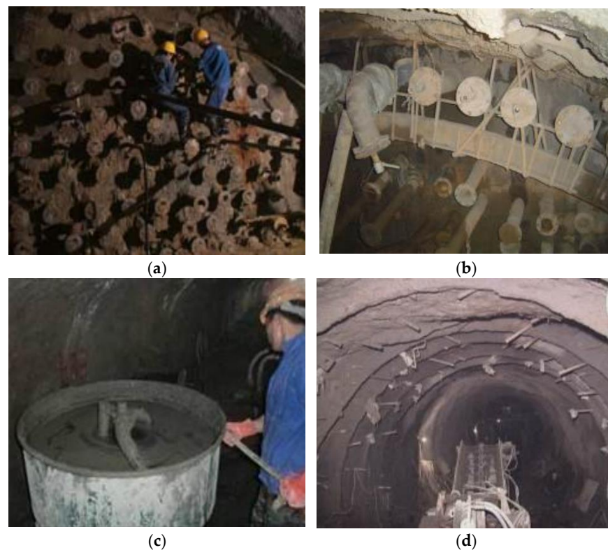
Figure 19. Processes of composite grouting [109]. (a) Advanced curtain grouting, (b) secondary reinforcement grouting, (c) localized infill grouting, (d) radial grouting.
