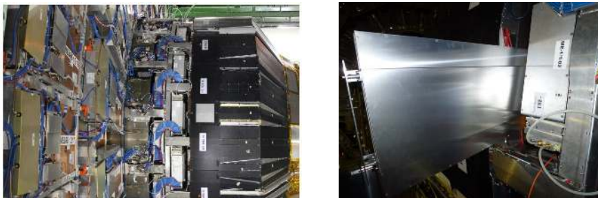
Figure 7. Left: location of the GE1/1 slots in the Muon endcap nose. Right: insertion of the dummy chambers.
