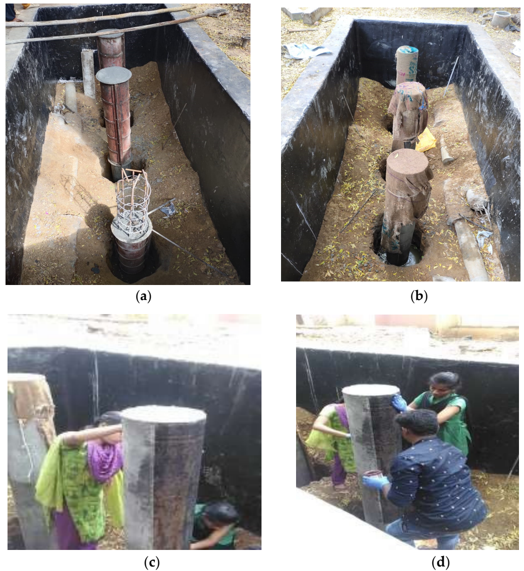
Figure 5. Casting of the FRP-wrapped piles: (a) placement of the reinforcement and concreting; (b) curing with wet gunny bags; (c) FRP wrapping; (d) coating of the epoxy above the FRP.
