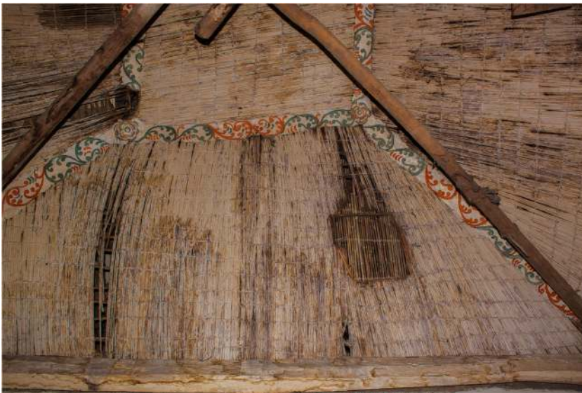
Fig. 7. Cuan net as part of the roof in a sixteenth-century house (Author's image)
