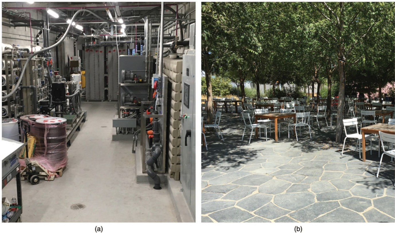
Fig. 4. (Color) Facebook's nonpotable reuse system (a) comprises microscreening, membrane bioreactors, reverse osmosis, and UV disinfection with chloramine and mineral adjustment; (b) The system is designed for 61,000 \text{ m}^3/\text{yr} (16 million gal./year) for irrigation of 5.3 ha (13 acres) of rooftop gardens and gathering spaces. This is an example of distributed water reuse, which is gaining popularity at large tech campuses and office buildings in California. (Images by authors.)
