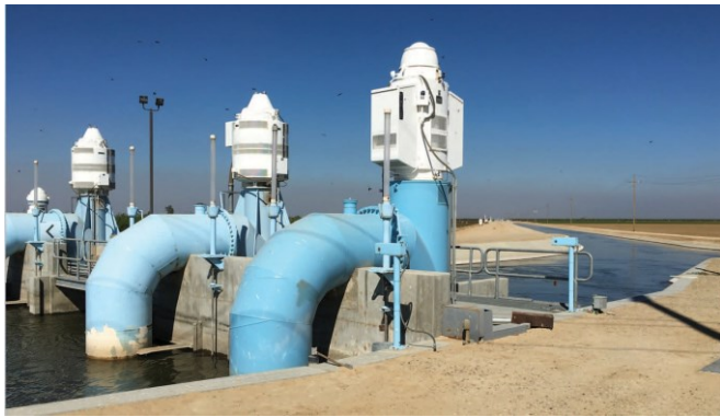
Fig. 6. (Color) Water banking facilities at the Semitropic Water Storage District allow water storage in Kern County, CA, and reverse flow of stored water back to the California Aqueduct. (Image by authors.)
