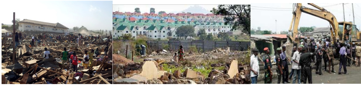
Figure 3. Sites of demolished illegal settlements in Apo Mechanic Village (left) and Mpape Satellite Town (middle and right), FCC, Abuja, Nigeria
