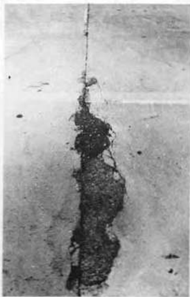
Figure 37. Knightstown Bridge - Progressive Failure of the Male Portion of the Joint. See Figure #36 for Location.
