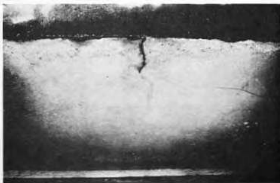
Figure #31. Area ① - One 3/4" diameter bolt broken, one tie-down clip missing; and one tie-down clip broken (See Figure #30 and Table 2).
