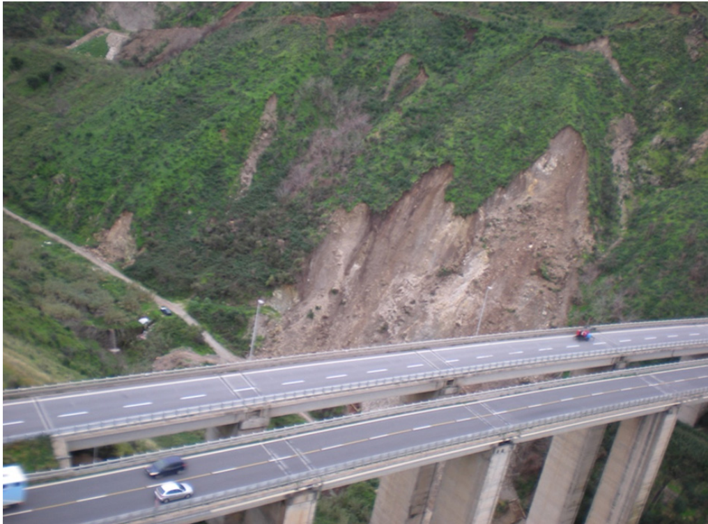
Fig. 2. Picture of Santa Trada landslide nearby the viaduct of the A3 motorway.
