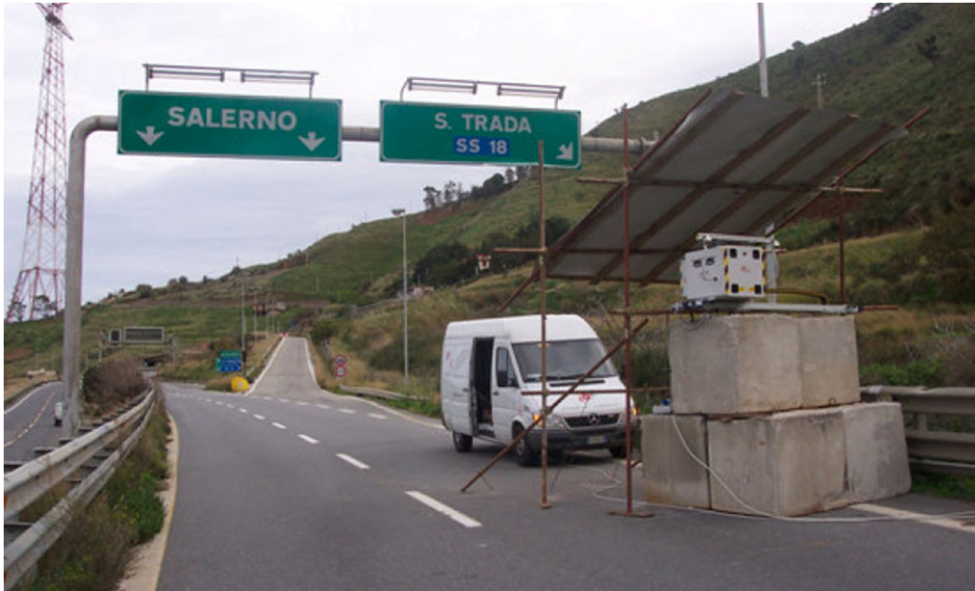
Fig. 4. Photograph of the GB-InSAR system installed on the motorway nearby Santa Trada.
