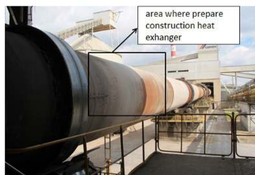
Figure 4. Rotary boiler number 4
