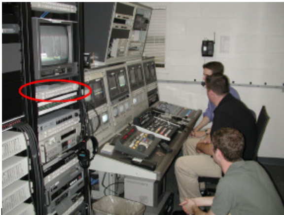
Figure 2 The DLPL control room following the 2004 renovation. The encircled area shows one of the routing switchers that provide a higher level of flexibility than had earlier been possible through the use of patch cords and similar temporary measures.
