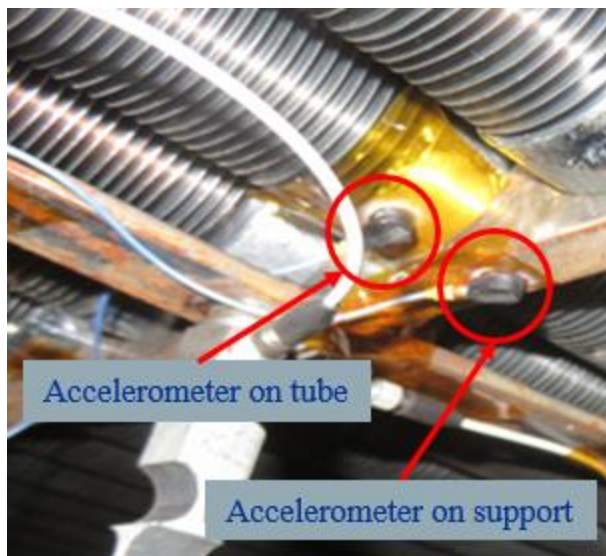
Figure 3. Select Supports Instrumented Both on and Adjacent to a Single tube
