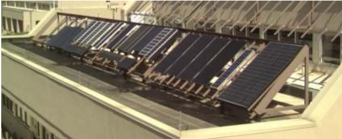
Figure 4-1. PV Modules on the PERT Rack at NREL's Outdoor Test Facility.
