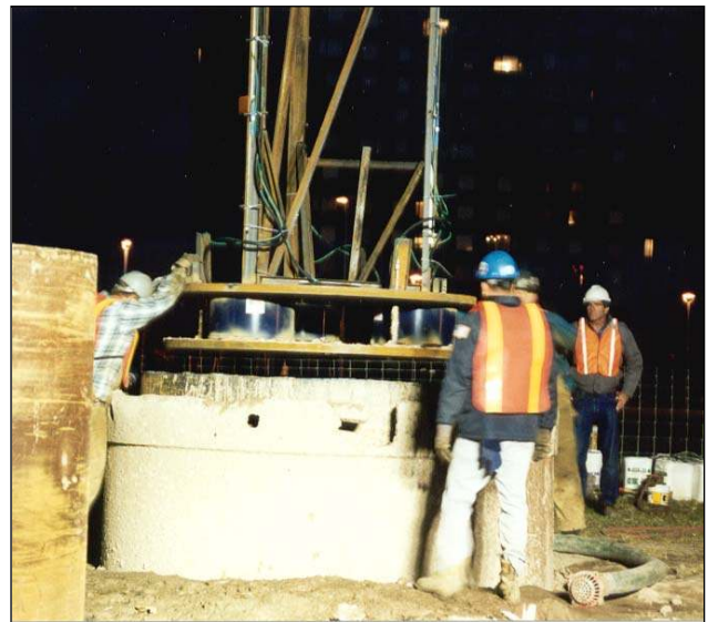
Photo 1.4. – The O-Cell assembly, complete with Instrumentation being lowered to the bottom of the prepared Drilled Shaft (before concreting)
