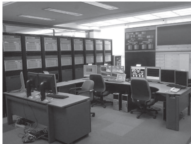
FIGURE 10. RTDS system in EHV power transmission company, CSG.
