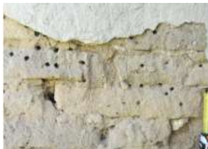
Figure 1. Exterior façade of a Caramel dwelling in Pinhal Novo, showing lack of protective render and degradation of adobe, by weathering and insects, showing the importance of a protective render.
