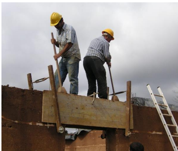
Figure 1 – Vernacular rammed earth formwork and manual compaction applied in a contemporary construction in Cercal, Alentejo, Portugal
