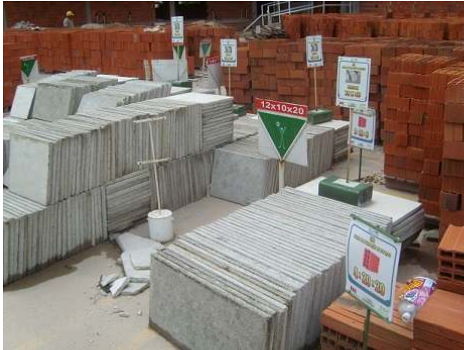
Figure 4. 5S Signs and kanban cards for material stock location standardisation and replenishment: Visual Management for process transparency and discipline
