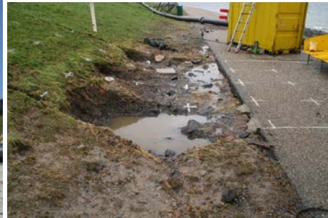
Figure 3. Damage caused by wave run-up simulation.
