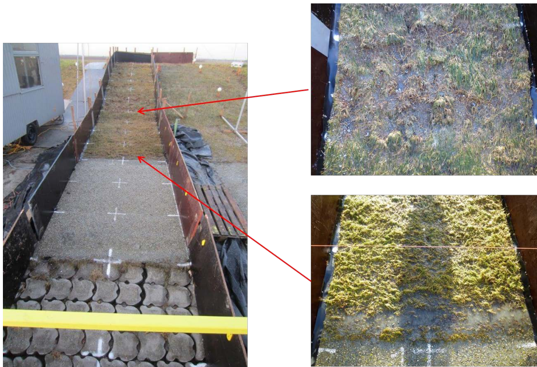
Figure 10. Damage to the transitions after test 1, showing hardly damage to initial damage
