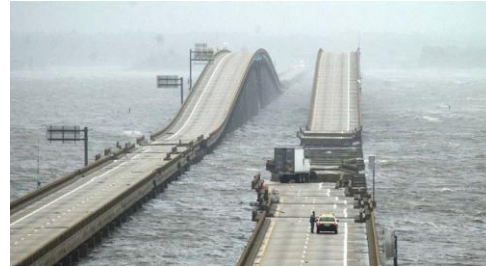
Figure 3. I-10 Bridge over Escambia Bay, FL after Hurricane Ivan.
