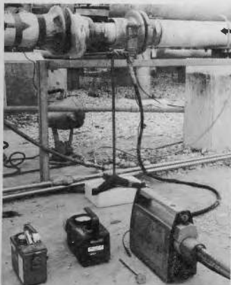
FIGURE 31 - FIELD RADIOGRAPHIC INSPECTION OF AN INVAR PIPE WELD IN VACUUM JACKETED PIPING
