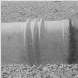
FIGURE 29 - FATIGUE CRACK IN THE CONVOLUTE OF AN EXPANSION BELLWS IN A VJ PIPE
