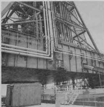
FIGURE 28 - VACUUM JACKETED PIPING INSTALLED AT THE BASE OF A MOBILE LAUNCHER
