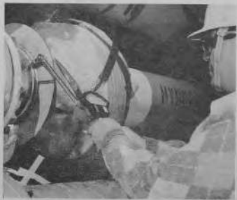
FIGURE 35 - INSPECTOR CHECKING THE INTERPASS TEMPERATURE ON A WELD IN VACUUM JACKETED PIPING
