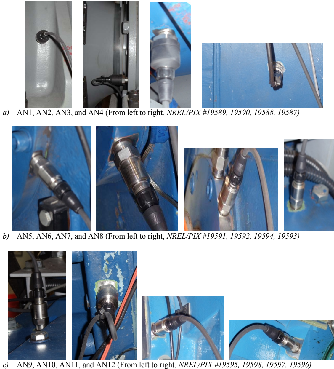
Figure 2.8. Physical sensor installation
