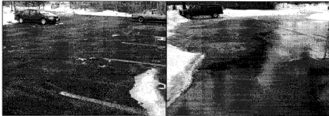
Figure 18: Instantaneous pavement conditions after freezing-rain: PA vs. DMA (1PM on 2/2/08) (18a) PA (left); (18b) DMA (right)
